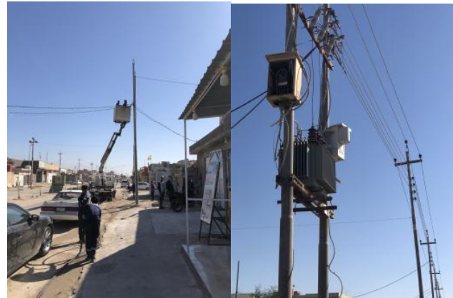
Poor Performance Transformers and a Part of the Maintenance Work in the City in 2021
